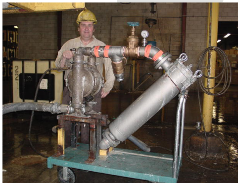
Closed-system Product Filtration that reduces product loss and sewer use bylaw pollutants, resulting in significant cost savings.
